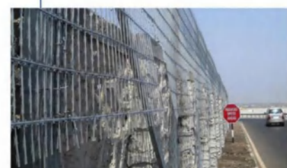
For highway protection
