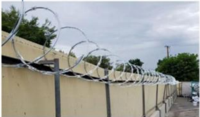
For factory isolation & protection
